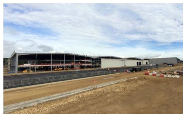
Hitachi's new plant at Newton Aycliffe is presently under construction. The £82m investment will see the assembly of nearly 900 new train carriages with the creation of 730 jobs.
