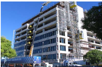
Construction of the new SAPOL headquarters at 100 Angas Street is due for completion in late 2011.
