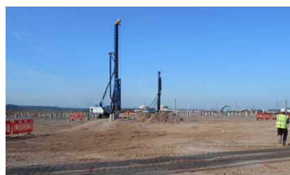
Farmfoods new chilled and frozen RDC at Central Park, Bristol is now under construction. The developer is Severnside Distribution Land & Roxhill.
