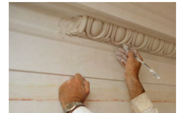
An architectural restorer carefully reworks carved plaster Ionic 'egg and dart' detailing
